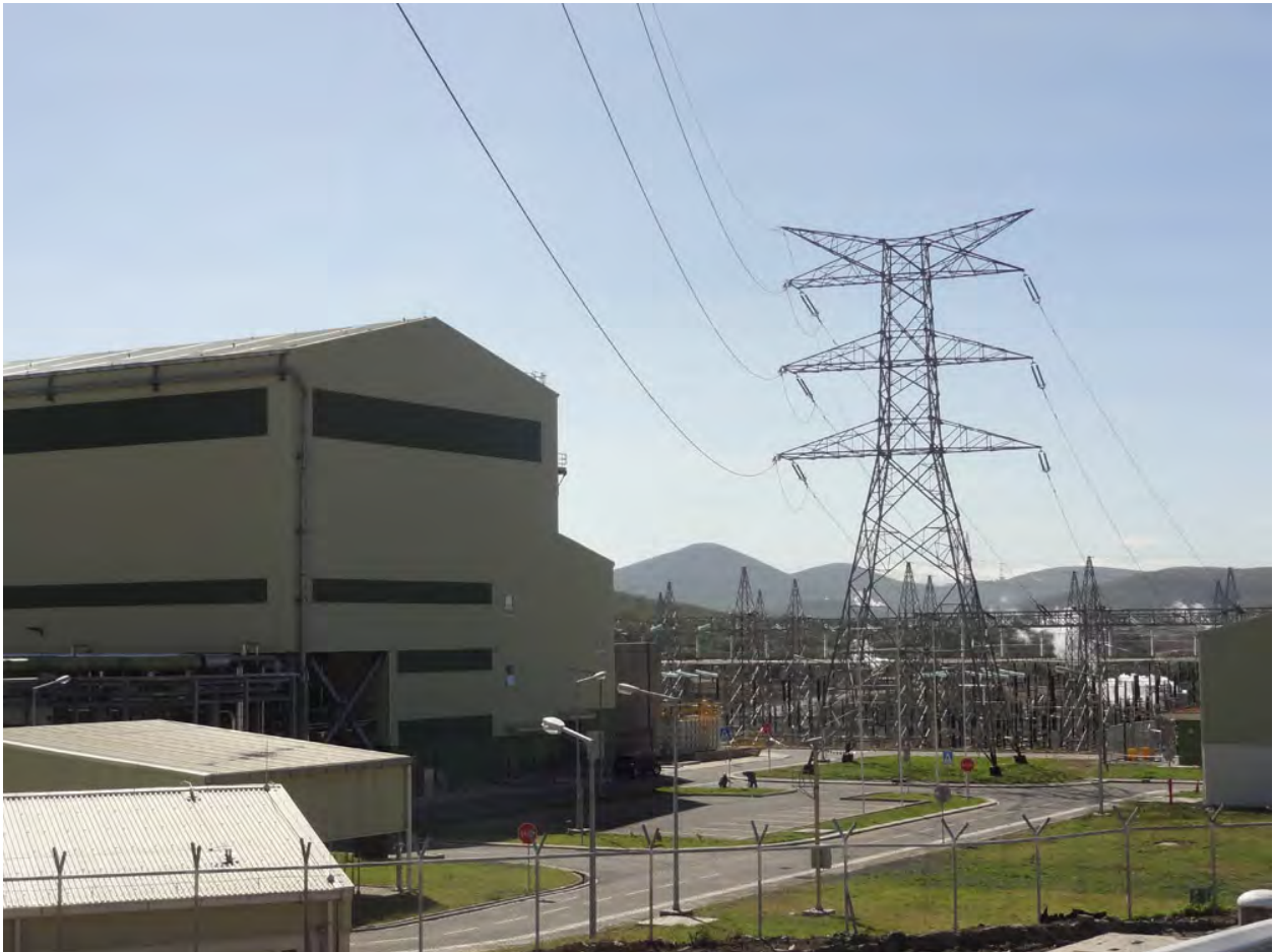
“Geothermal power station Olkaria I (Kenya)” (© Jeanette Schade)
