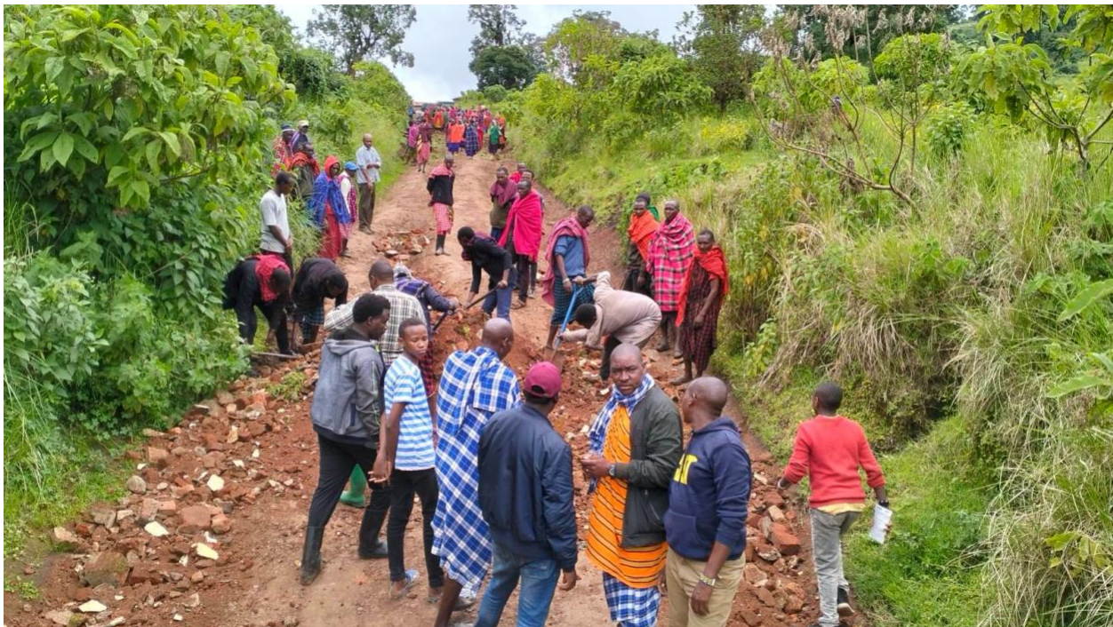
Residents joined forces to repair roads to Olorobi Primary School and Oloirobi Health Centre
